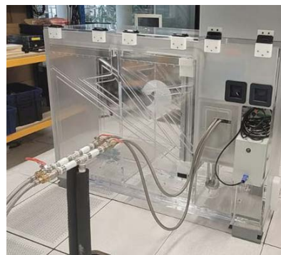
Liquid connection to the datacenter sealed water loop
