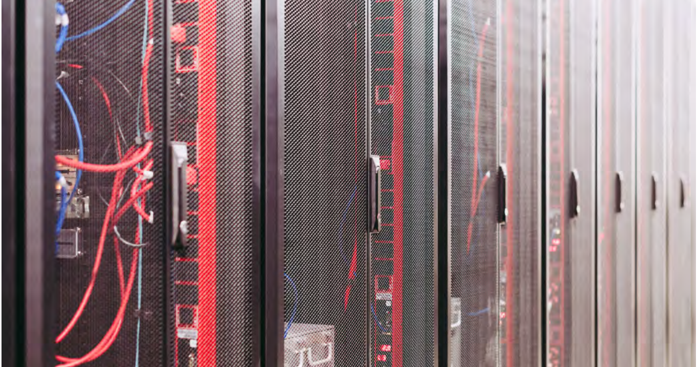
Data Centers and their cooling consume huge amounts of energy and also lead to E-waste. We need Data Centers and we need to do better at how we maintain them.
